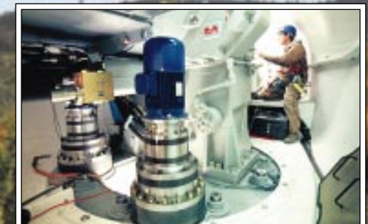
The nacelle provides a weather protected, enclosed and spacious environment for field personnel to perform service and maintenance work.
